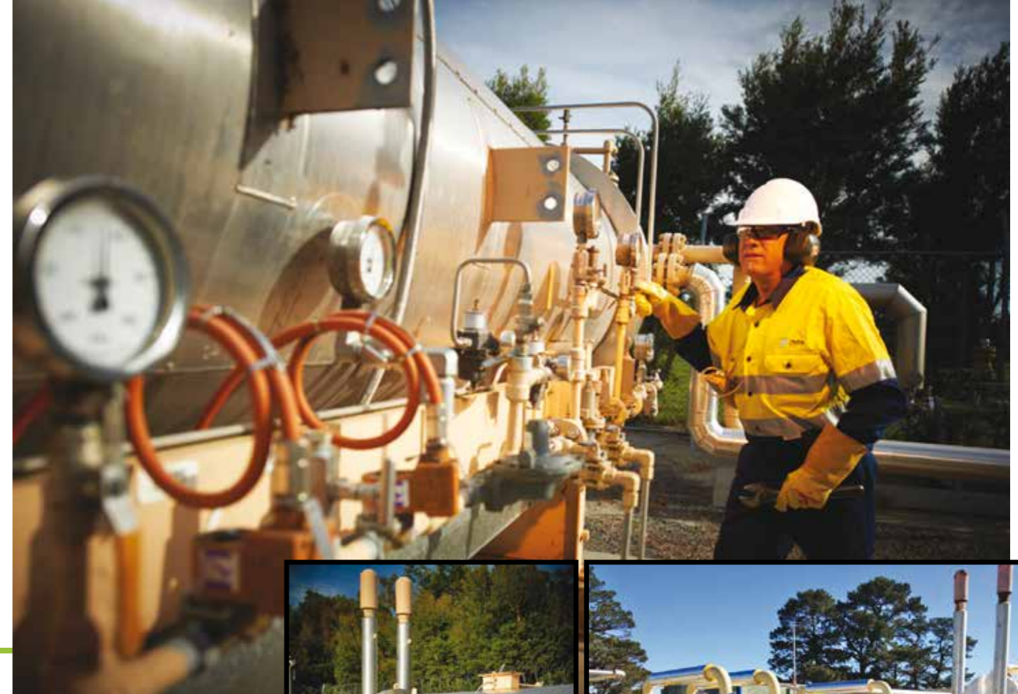
Top and left: A Zinfra employee working on gas pipelines. Right: The Fyshwick Trunk Receiving Station (TRS).
